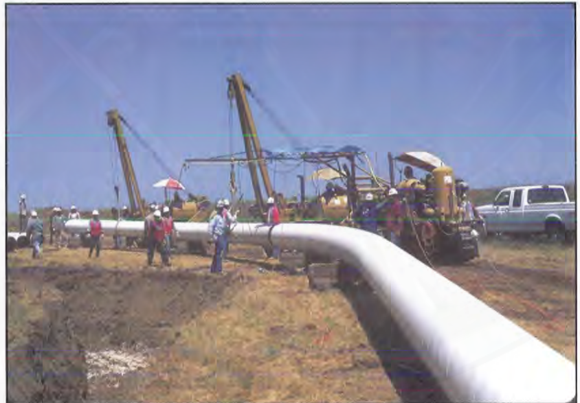
Figure 3. The 24 inch-diameter Fort Union Gas Gathering Pipeline, along with several other large pipelines, transport coalbed natural gas from the Powder River Coal Field.
