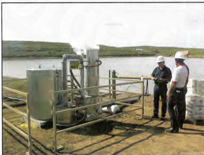
Figure 7. Harmon Model 30 amending CBNG production water in Pit Reservoir.
